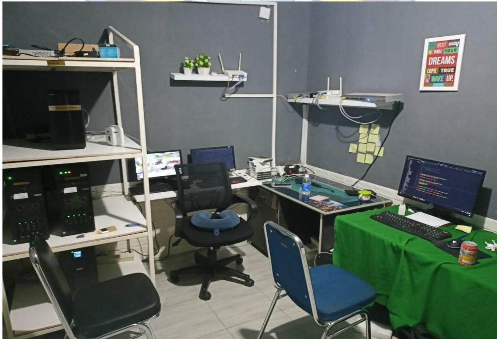
Ruang Admin Server
